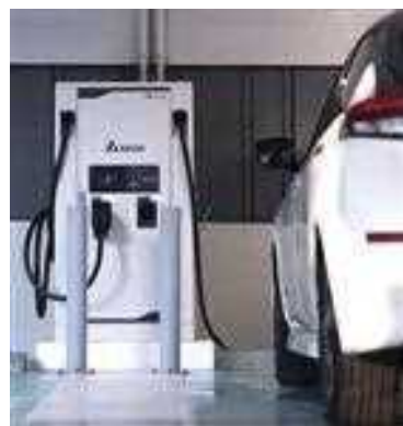
Photo: Delta Electronics Thailand.
