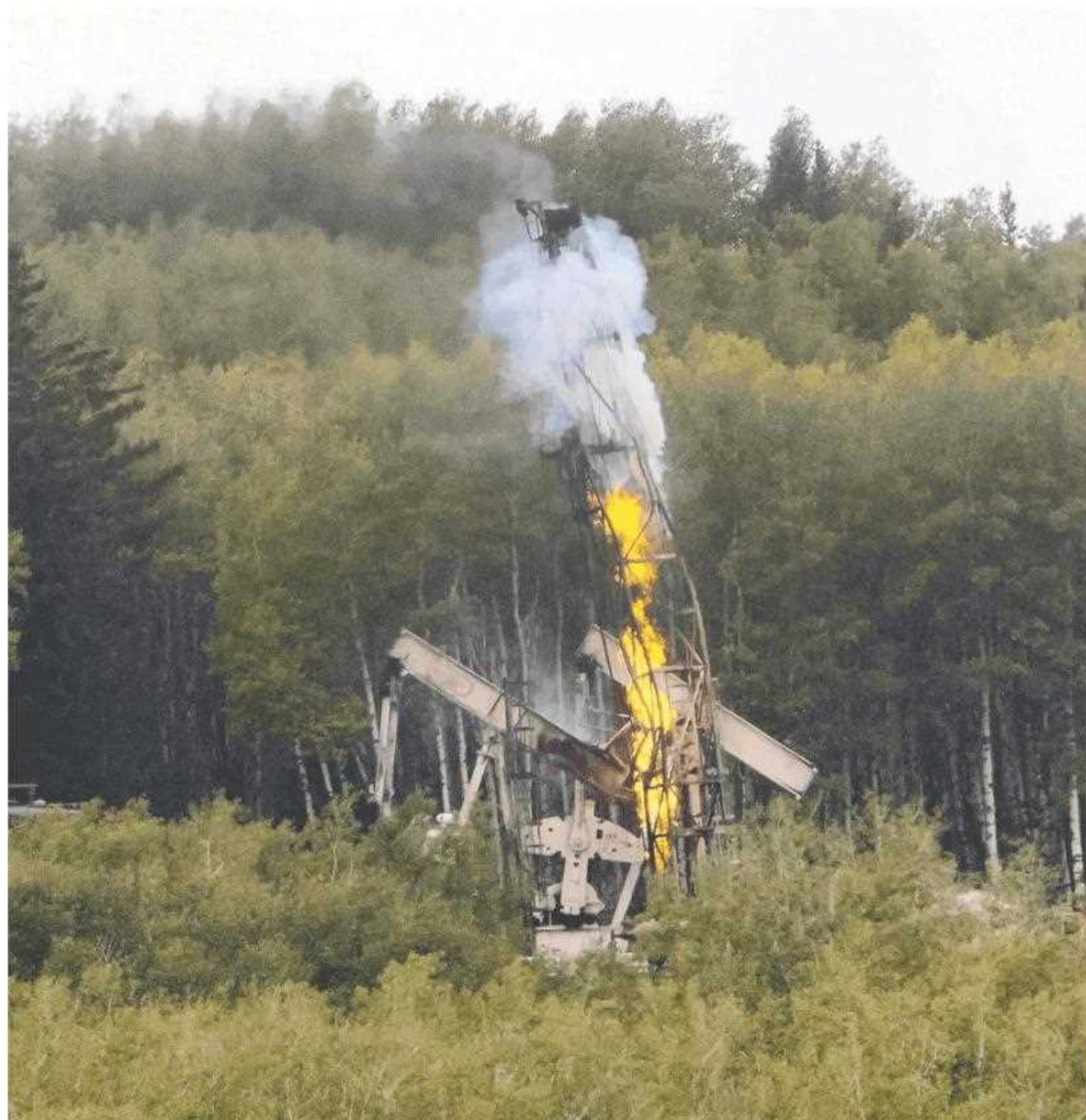
Five workers were hospitalized after an explosion at an oil well site north of Cochrane on Monday. Three of those people suffered life-threatening injuries, Alberta Health Services EMS said. DARREN MAKOWICHUK
