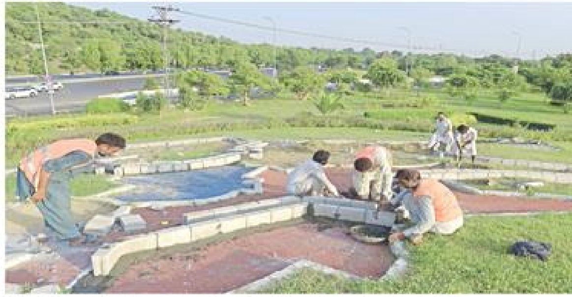
LABOURERS carry out renovation work on a greenbelt near Zero Point Interchange in Islamabad. — White Star
