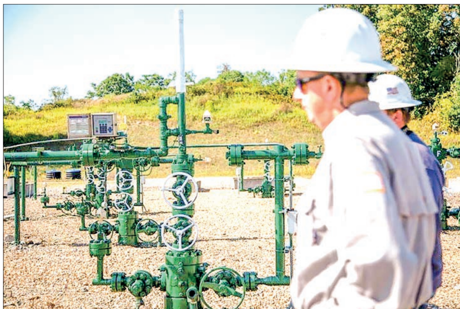
Diversified Energy employees stand by natural gas well in Franklin Township, Washington County, Pennsylvania. PHOTO: AFP
