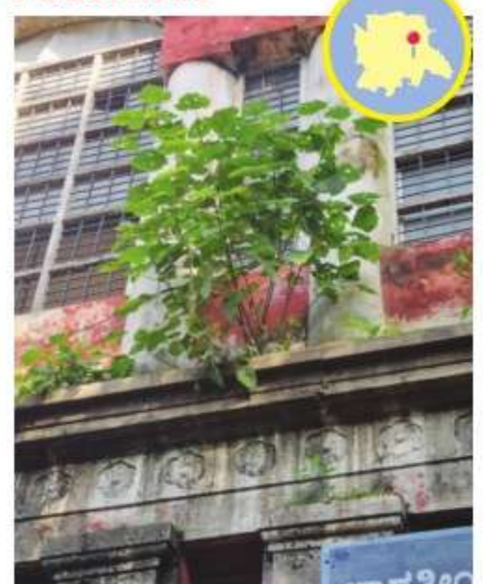
The Law College building on Palace Road, near Mysore Bank Circle, is in poor condition, highlighting an urgent need for maintenance and repairs.
