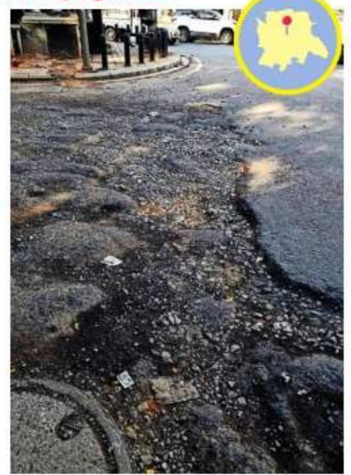
The area in front of Kaveri Bhavan near Kempegowda Road is marred by numerous potholes.
