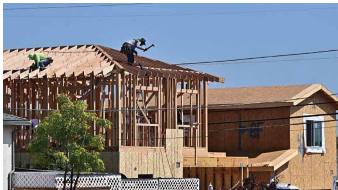
ALHAMBRA, US: Construction workers work on the roof of a house being built in Alhambra, California on Sept 23, 2024. — AFP
