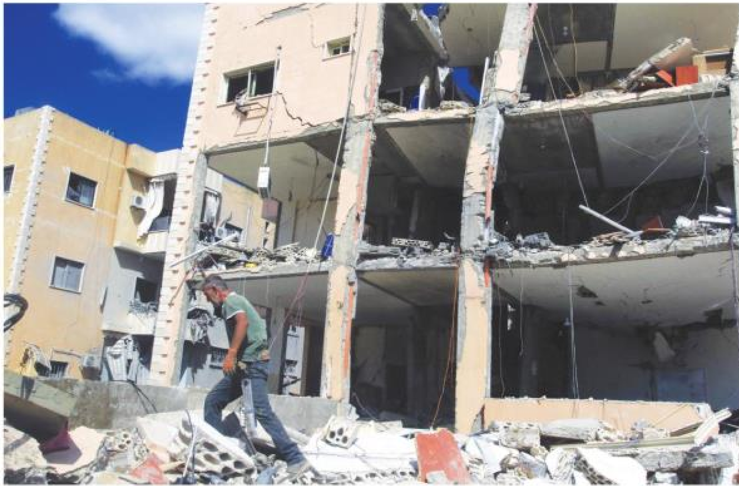
Several buildings were heavily damaged in Israeli strikes in Kfar Rumman near the southern Lebanese town of Nabatieh on Friday night. AFP
